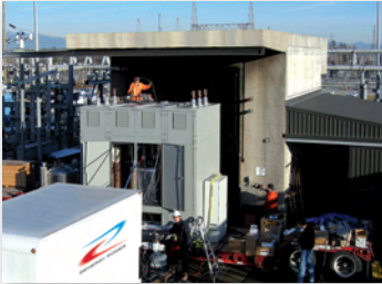
Fault Current Limiter Image Courtesy of Zenergy Power
