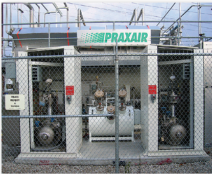
Two 1kW pulse tube cryocoolers installed at HTS cable site Image courtesy of Praxair, Inc.
