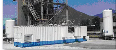
Small containerized cooling facility suitable for HTS cable Image courtesy of Air Liquide
